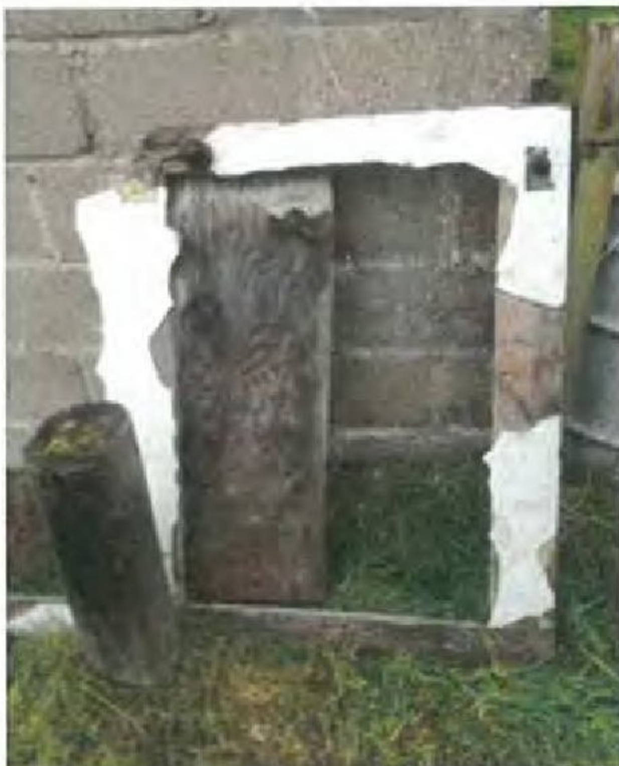
Figure 6. Door frame debris with asbestos cement sheeting attached
